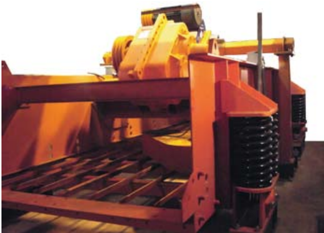
Fig. 21a Coal crusher shaft
