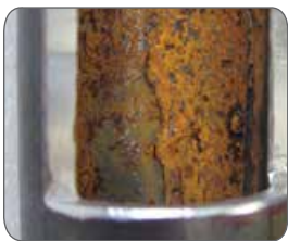
Atmospheric Dirt Rust Pipe scale
