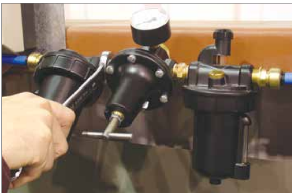
This makes maintenance more difficult
